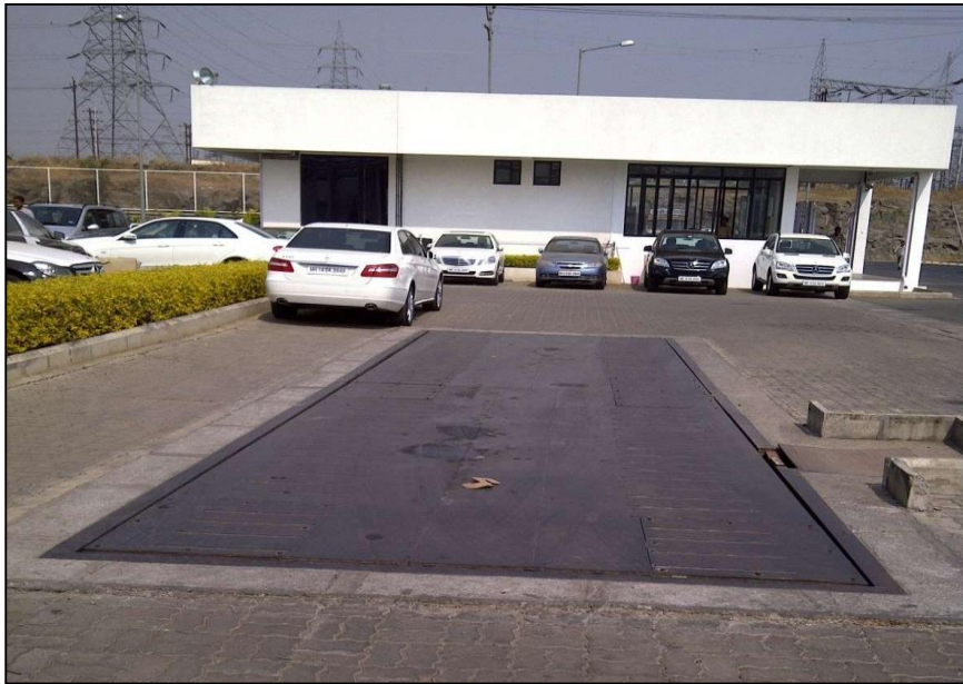
Pit Type Weighbridge
